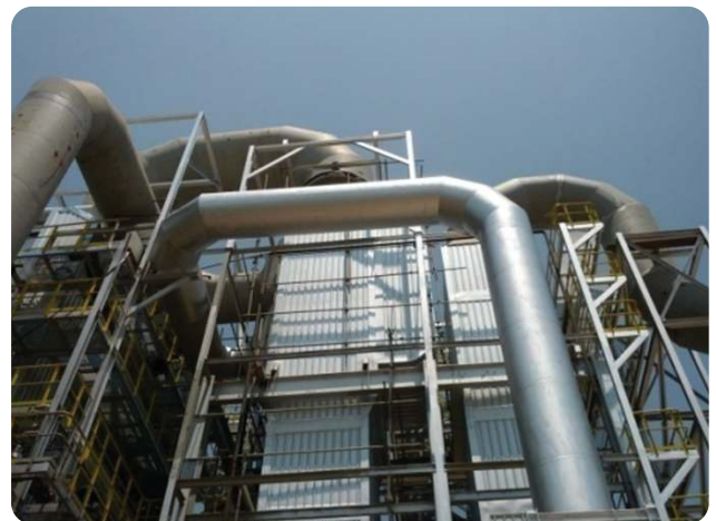
6.5 MW Empty Fruit Bunch/Palm Fiber Fired Power Plant, Surat Thani Province
