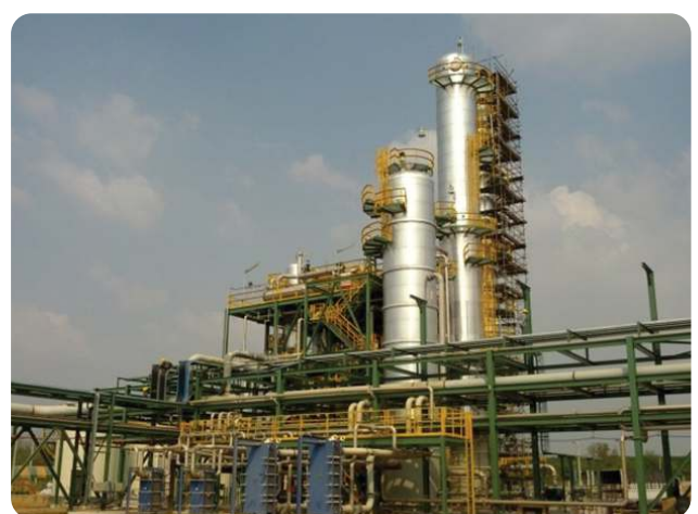
200,000 LPD Ethanol Distillation Plant, Chachoengsao Province
