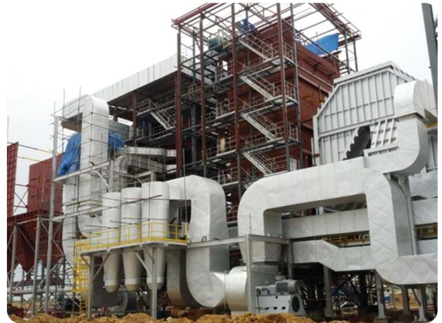
9.9 MW Wood Bark Fired Power Plant, Buriram Province
