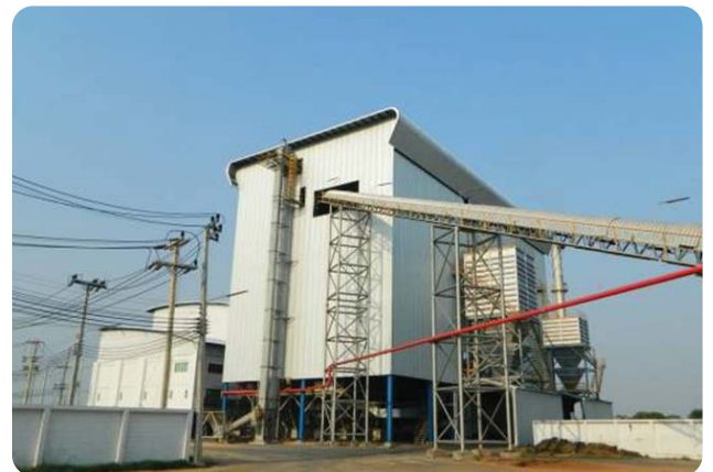
9.9 MW Rice Husk Fired Power Plant, Nakhon Ratchasima Province
