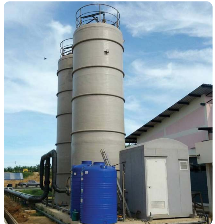
H 2 S Bio-Scrubber System, Tha Sae Cooperatives, Chumporn Province
